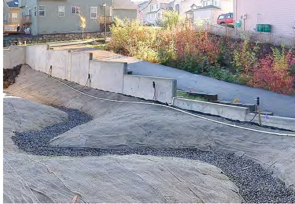
Figure 3: Bioswales for housing development. (Foreground is under construction and background is established)
