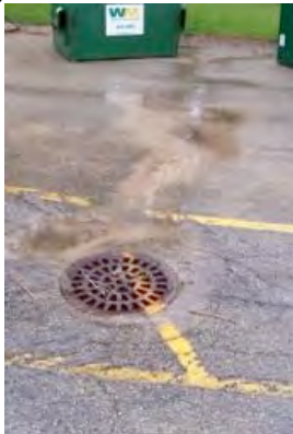
Figure 2: Rain water runoff
